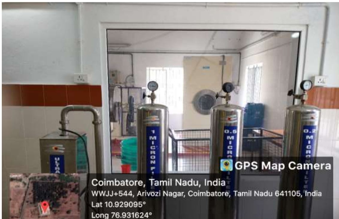
Filtration units inside RO plant
