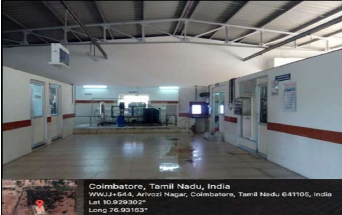
RO plant front view
