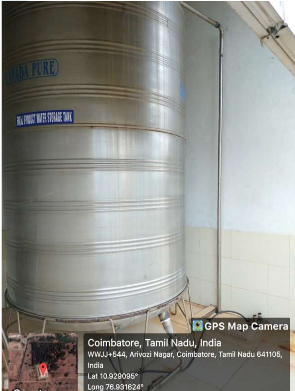
Filtered water storage unit
