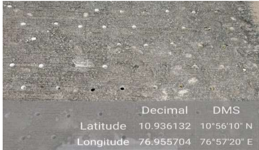
Perforated drain channel slabs (Close view)
