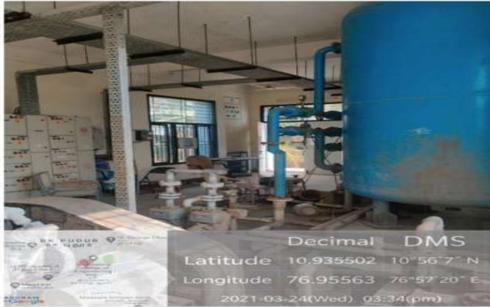
Secondary treatment units and treated water storage area
