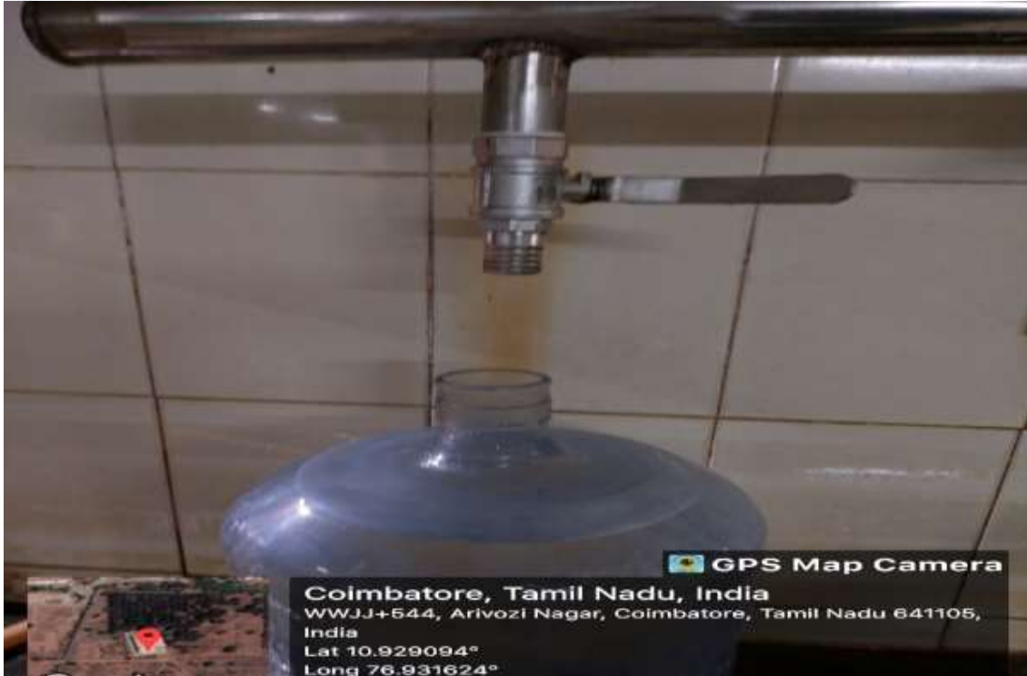
Filtered water to water cans for distribution
