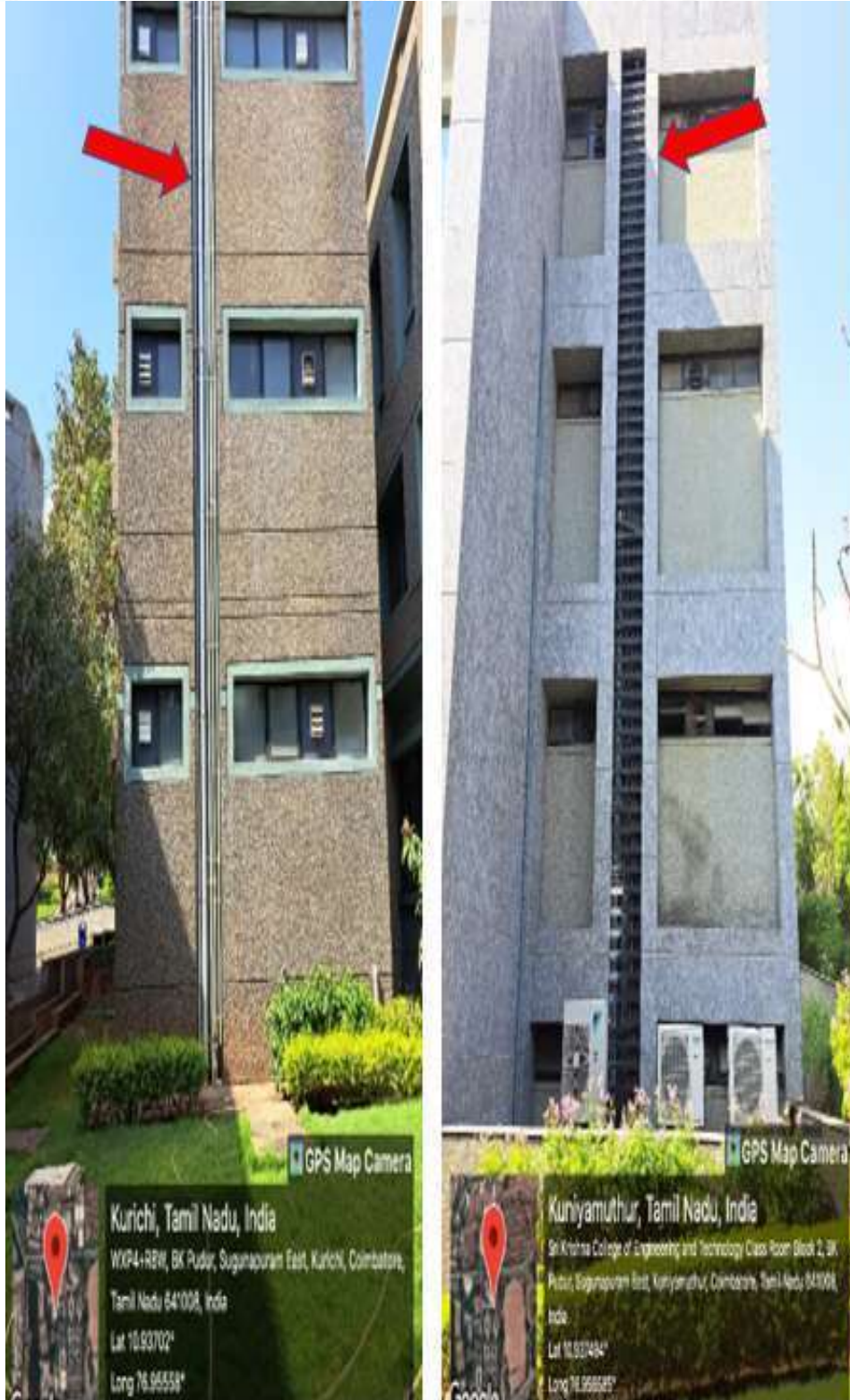
Distribution pipes in MCA block (Left side) and Admin block (right side)
