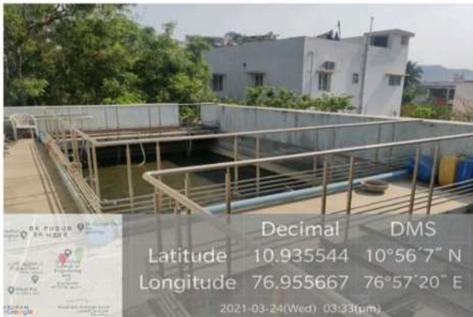
Primary treatment units
