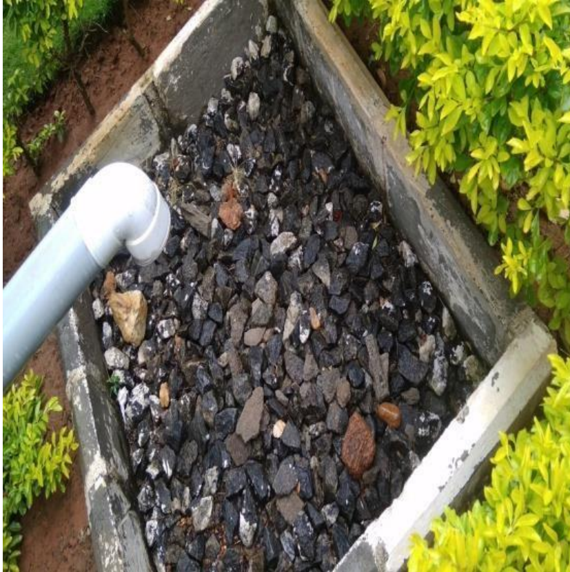
Rainwater Harvesting Pit
