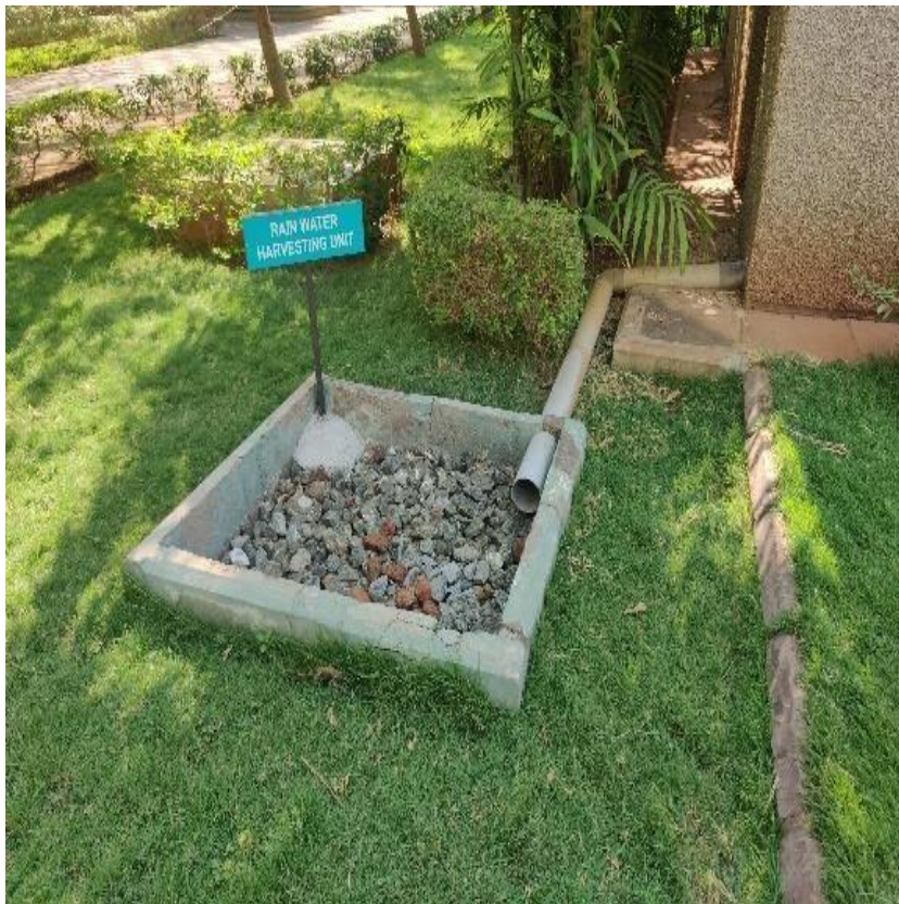
Rainwater Harvesting Pit
