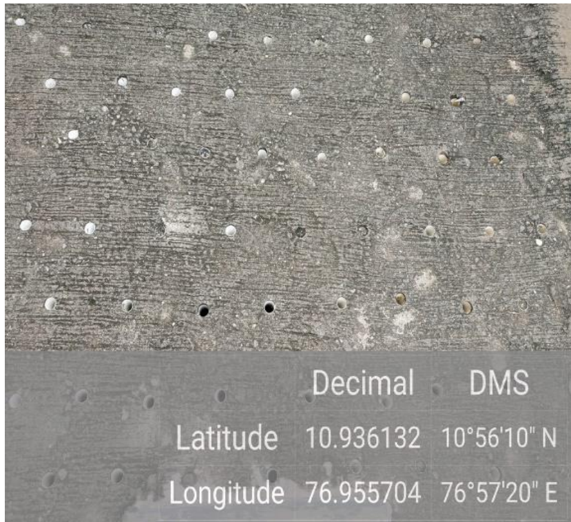
Perforated Drain Channel Slabs (Close view)
