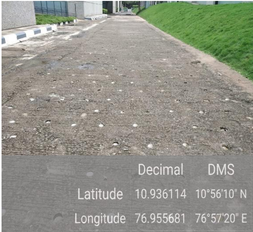
Perforated Drain Channel Slabs (Long view)
