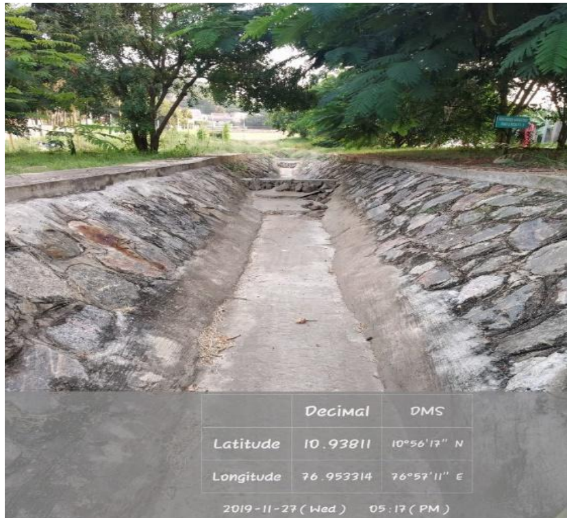
Percolation pits by deep bore holes (Dry Season)
