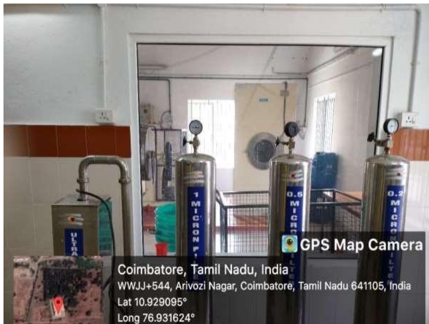
Filtration units inside RO plant
