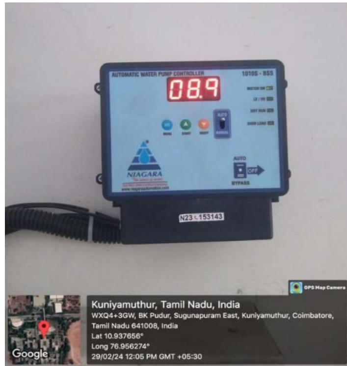
Automatic Water Pump Controller – Administrative Block
