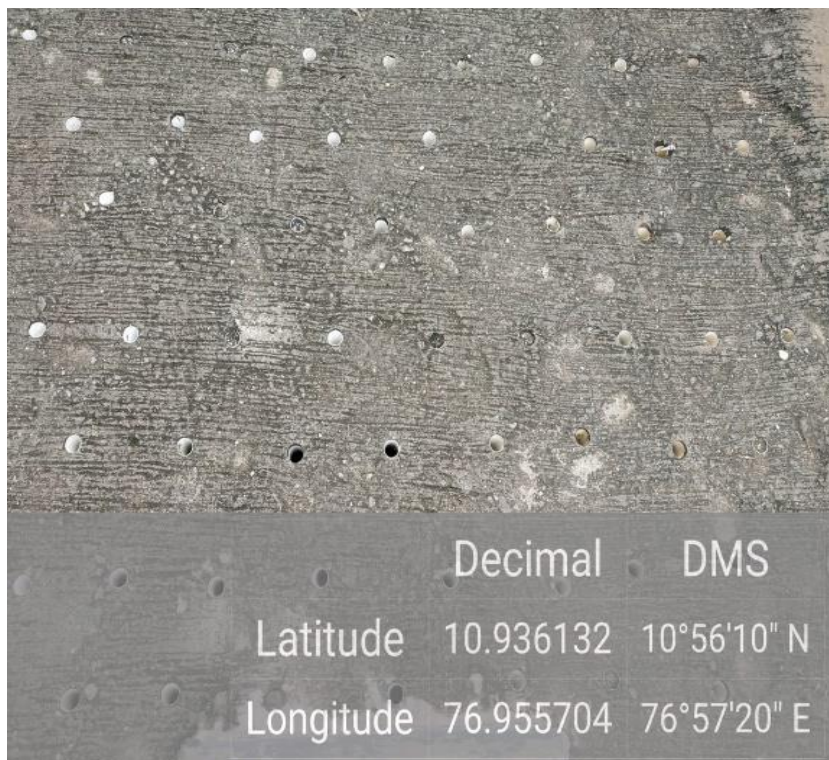
Perforated Drain Channel Slabs (Close view)
