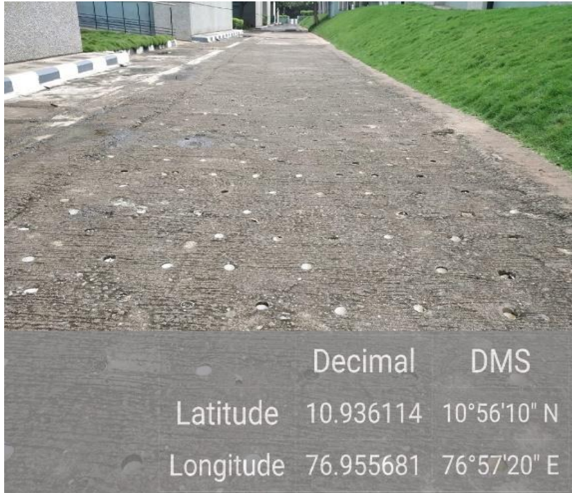
Perforated Drain Channel Slabs (Long view)
