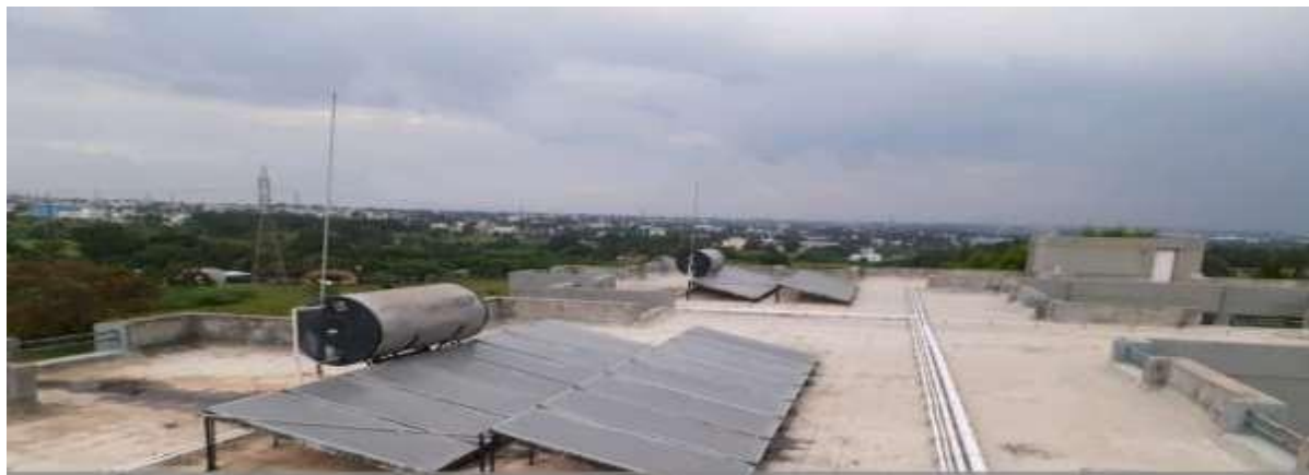
Solar water heater installed in Hall of Residence Women-'B1' Block 3000LPD with 5bar(kg/cm 2 )
