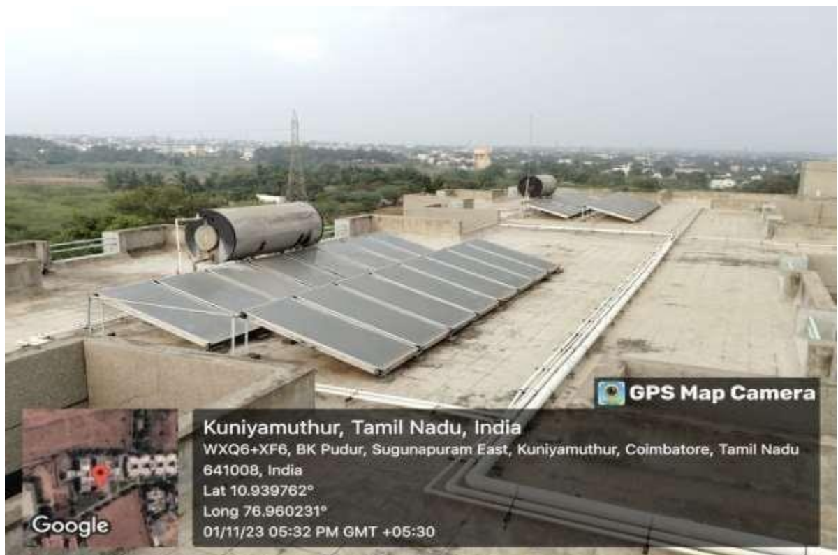
Solar water heater installed in Hall of Residence Men –‘B’ Block 3000LPD with 5bar(kg/cm 2 )
