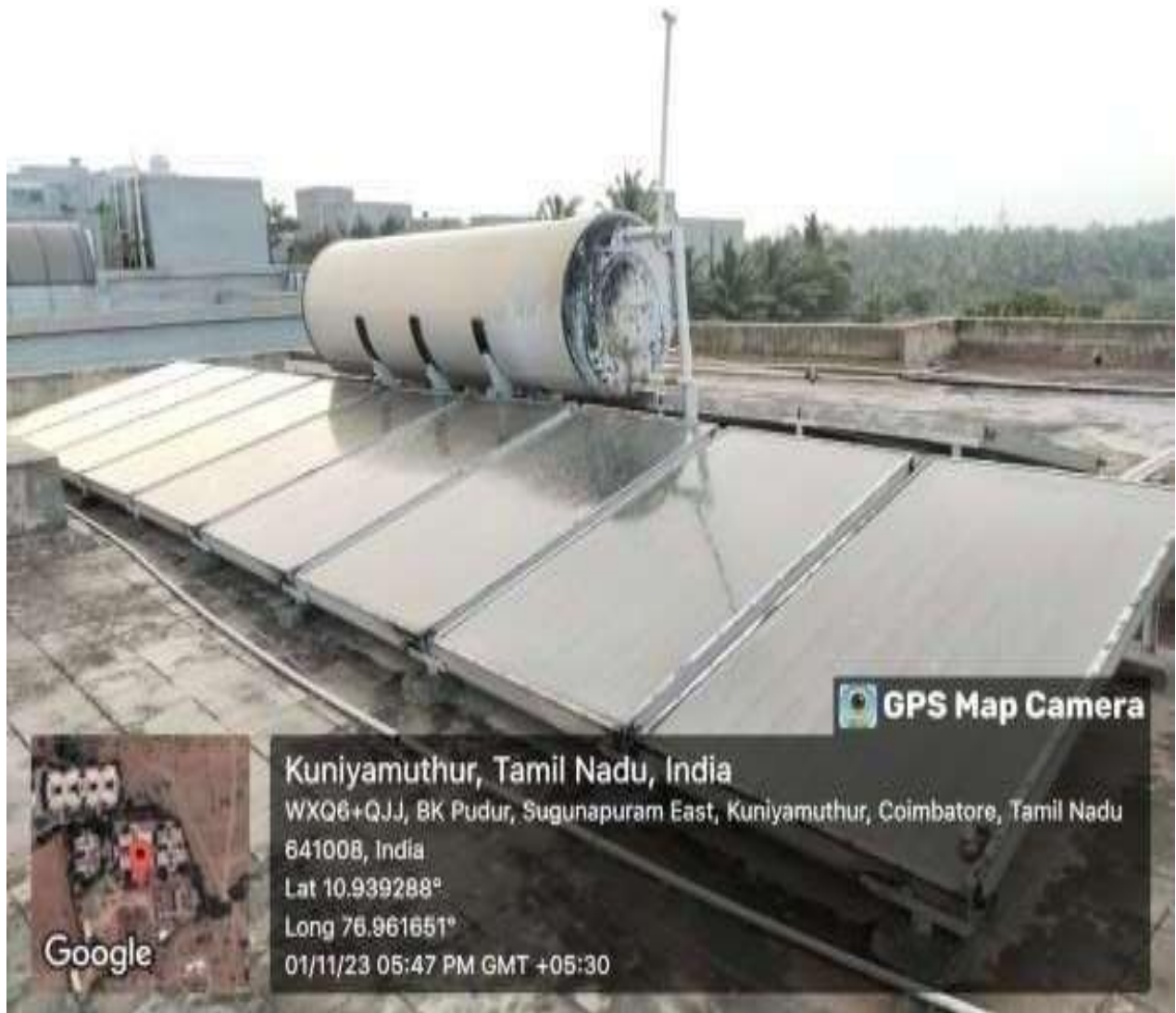
Solar water heater installed in Hall of Residence Men –‘E’ Block 3000LPD with 5bar(kg/cm 2 )
