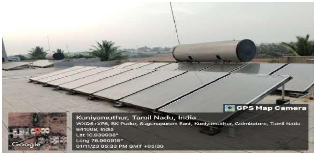
Solar water heater installed in Hall of Residence Men –‘A’ Block: 3000LPD with 5bar(kg/cm 2 )
