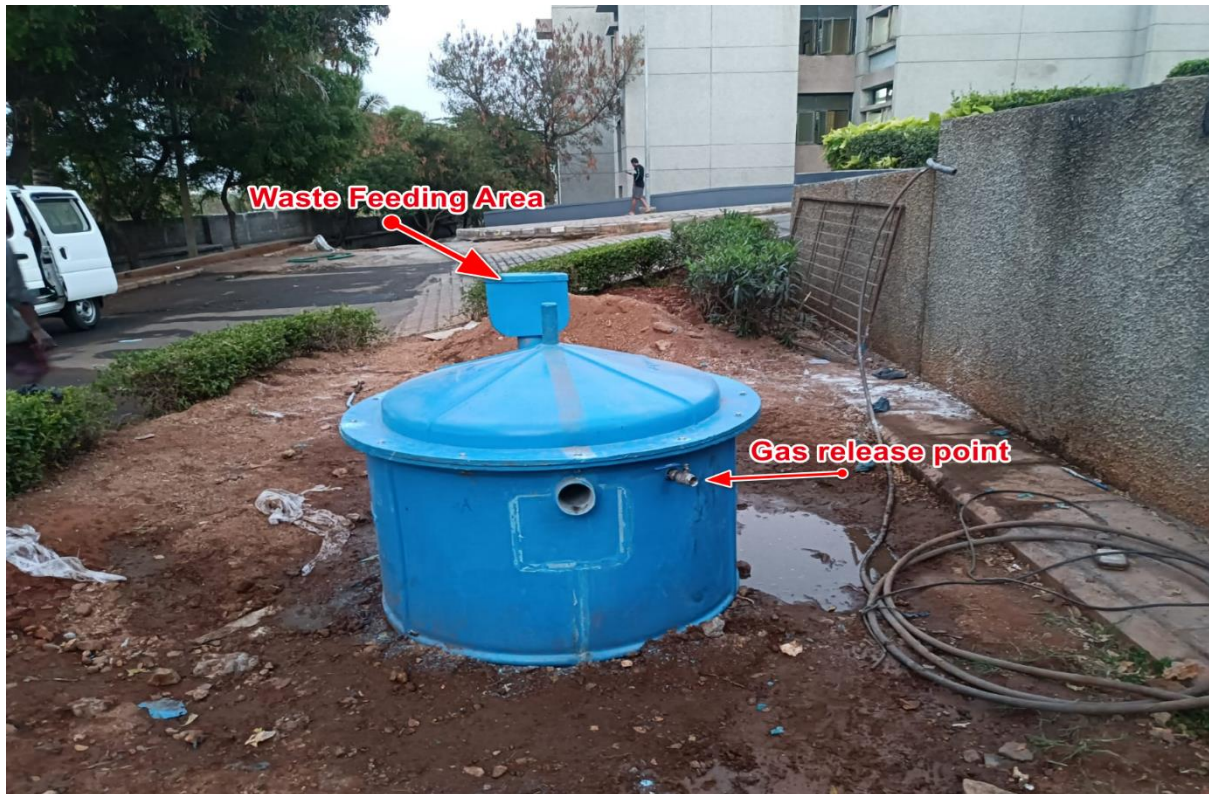
Biogas plant full setup
